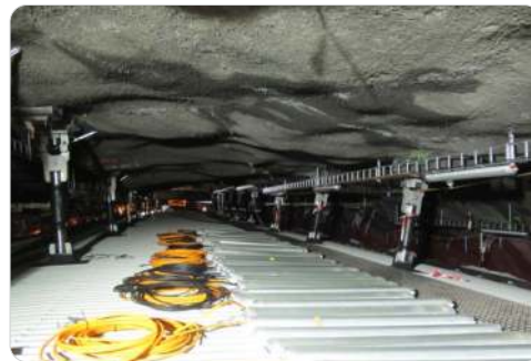
Dynamic hangers in Holmestrand train tunnel Picture courtesy of Sandvik Materials Technology
