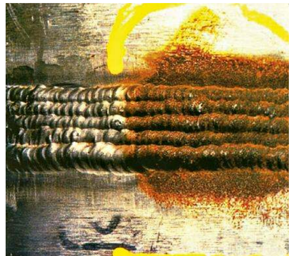
Carbon steel wire brushes used to “clean” stainless steel welds can produce discoloration and rust. Stainless steel wire brushes must be used. © Outokumpu Stainless
