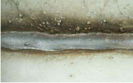
Weld spatter and an irregular weld bead should be avoided. © Outokumpu
