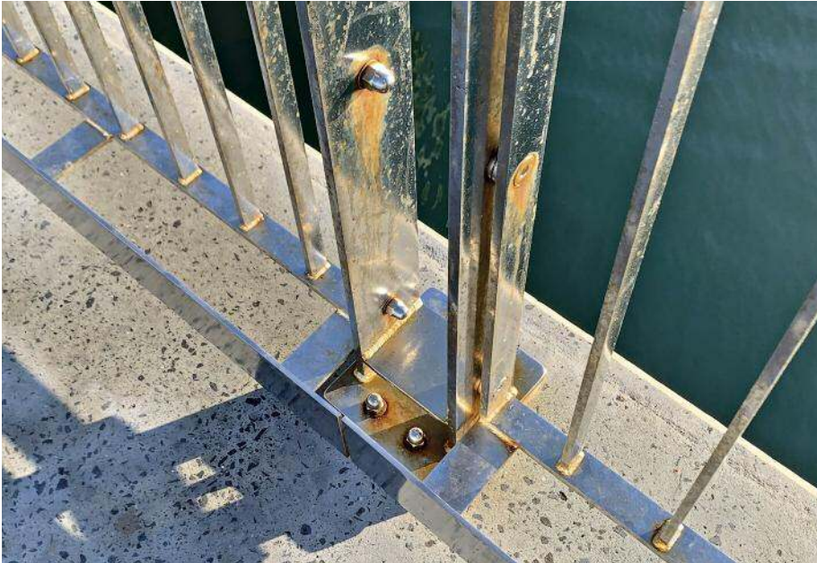
Crevice corrosion at the bolted connections of a hand rail exposed to seawater splashing. © Graham Sussex
