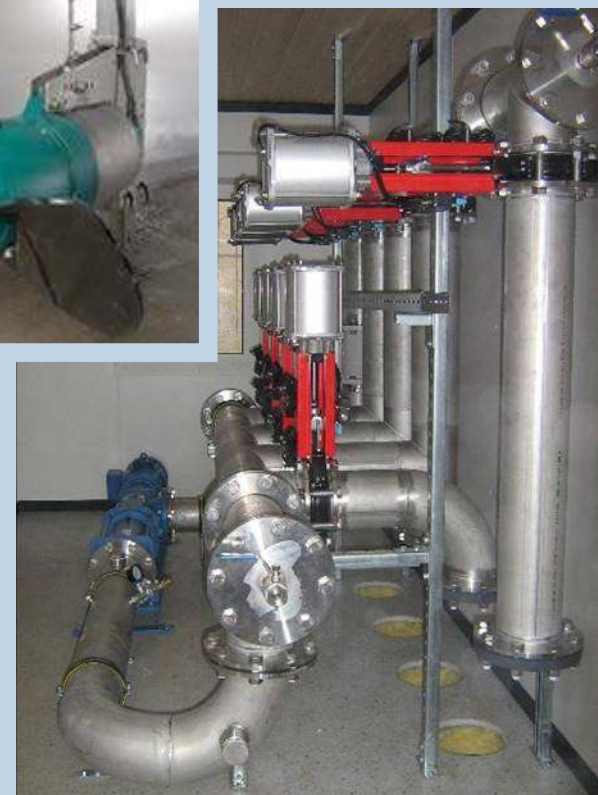
Screw pump with stainless steel piping
