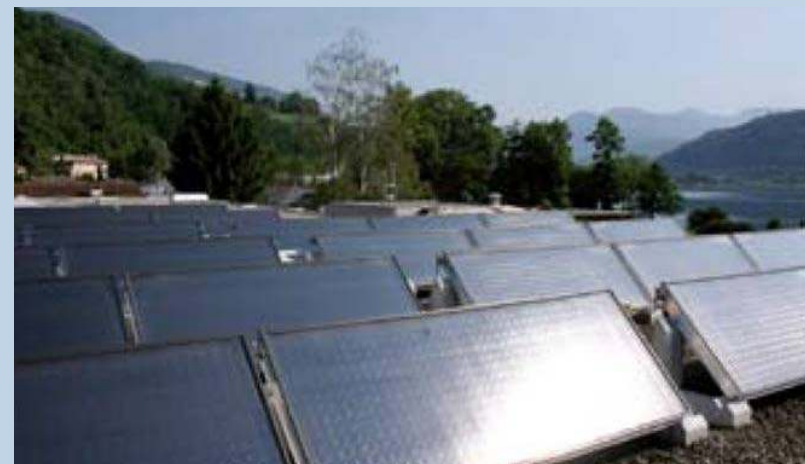
Solar panels with cushion absorbers
