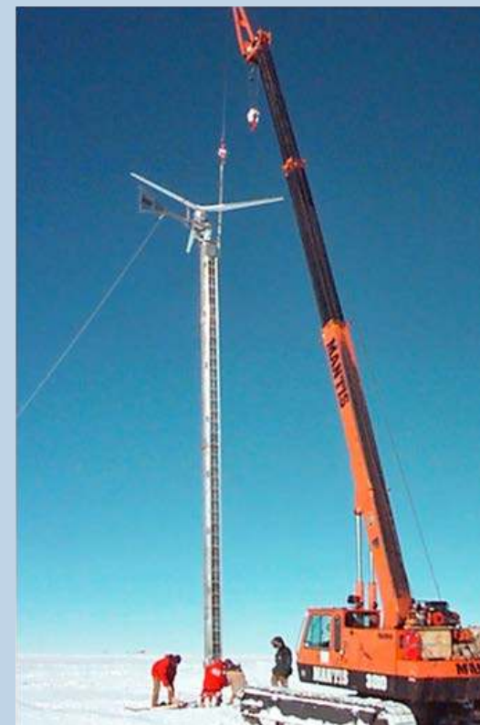
16 m tubular tower
