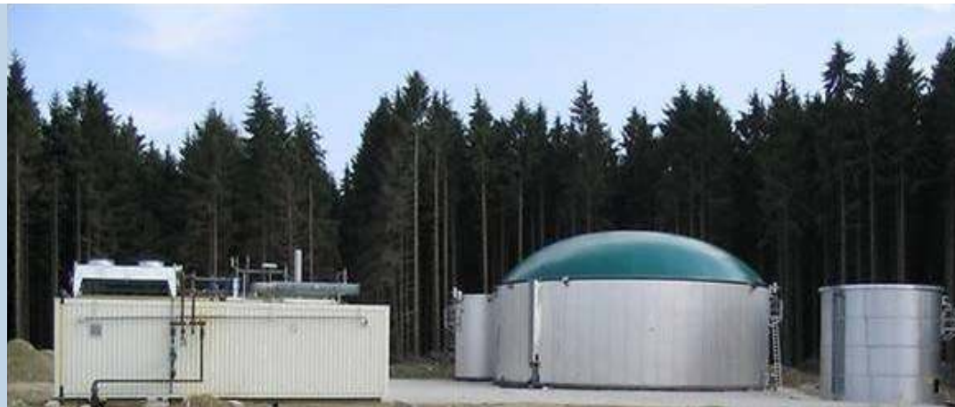
Frankfurt Hahn Airport's co-generation plant
