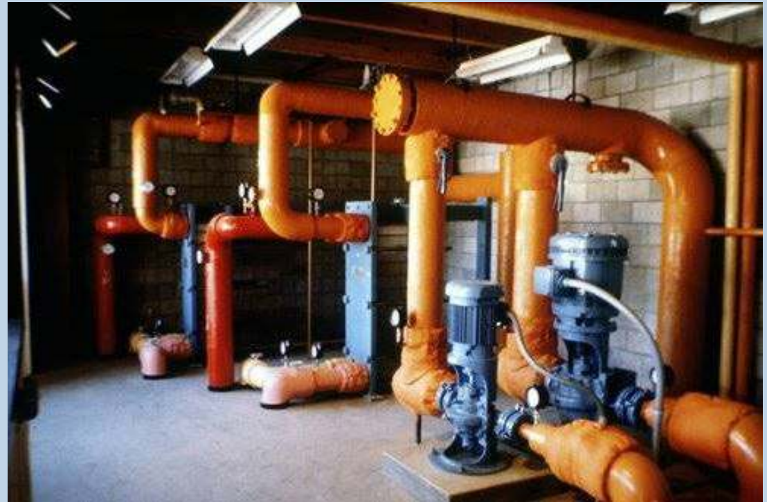
Heating exchangers and circulation pumps in a geothermal district heating system (Klamath Falls, USA)
