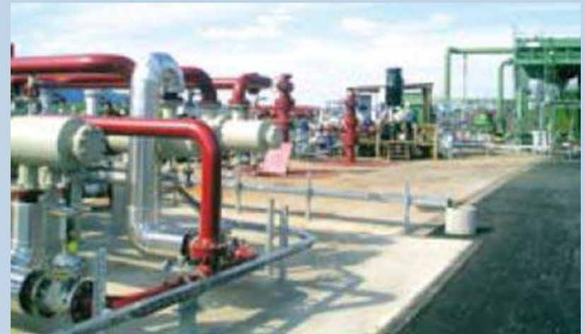
1.5 MW binary EGS power plant (Soultz-sous-Forêts, France)
