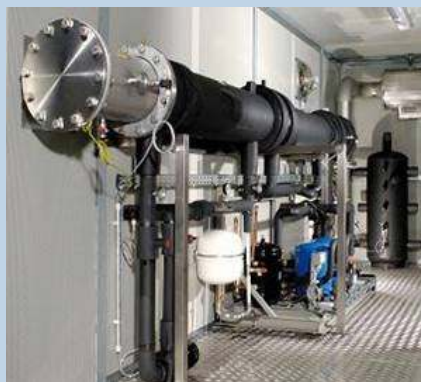
Biogas drying unit
